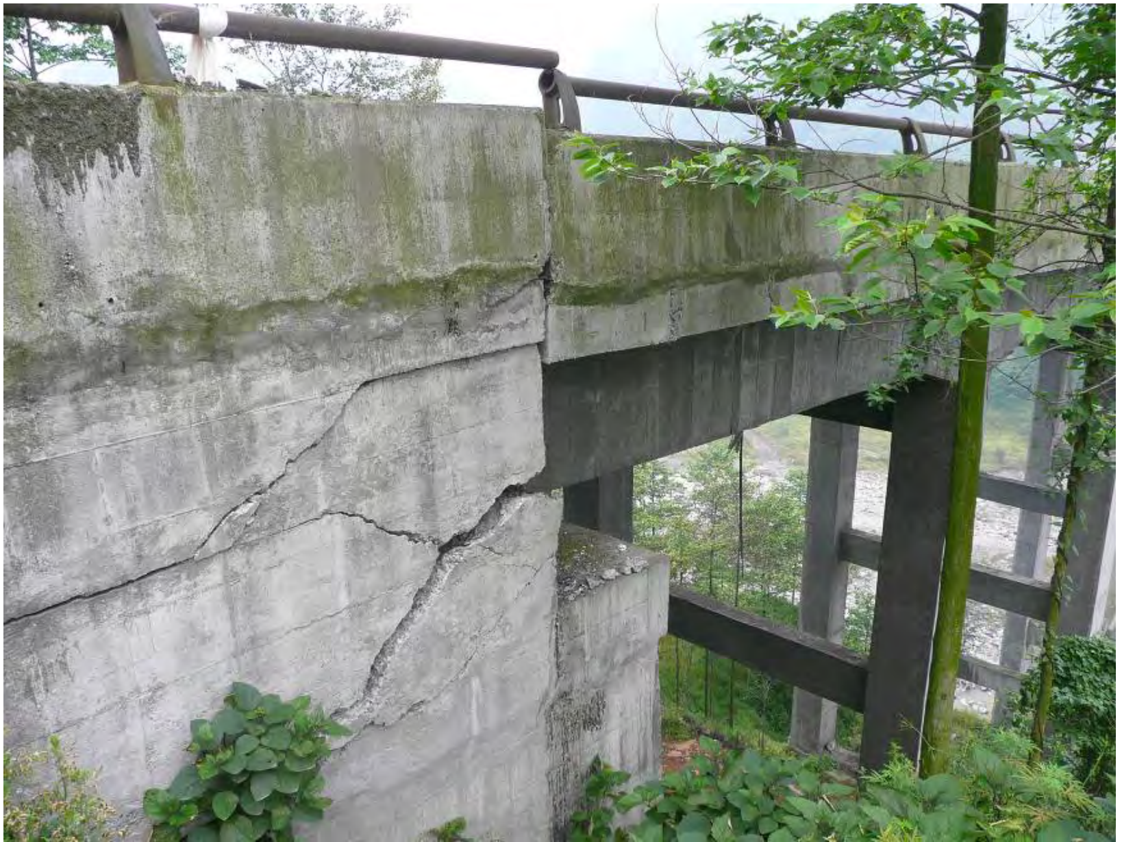
Crack in abutment
