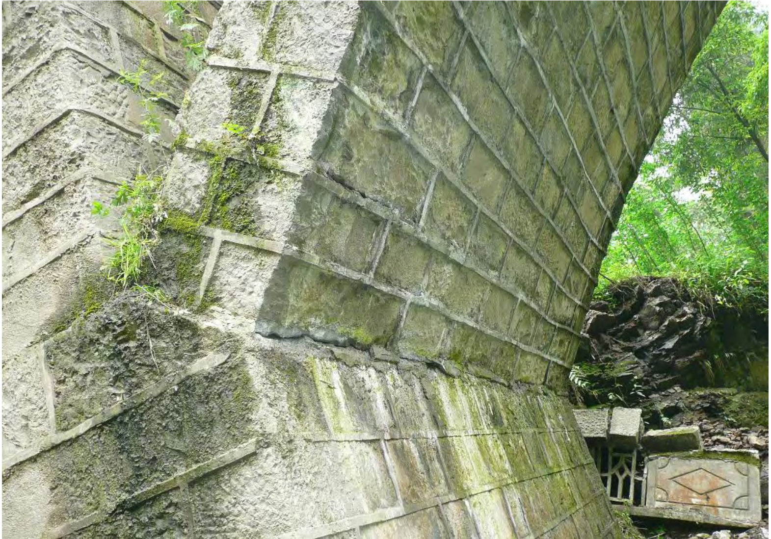
Showing cracks at the bottom of the arch
