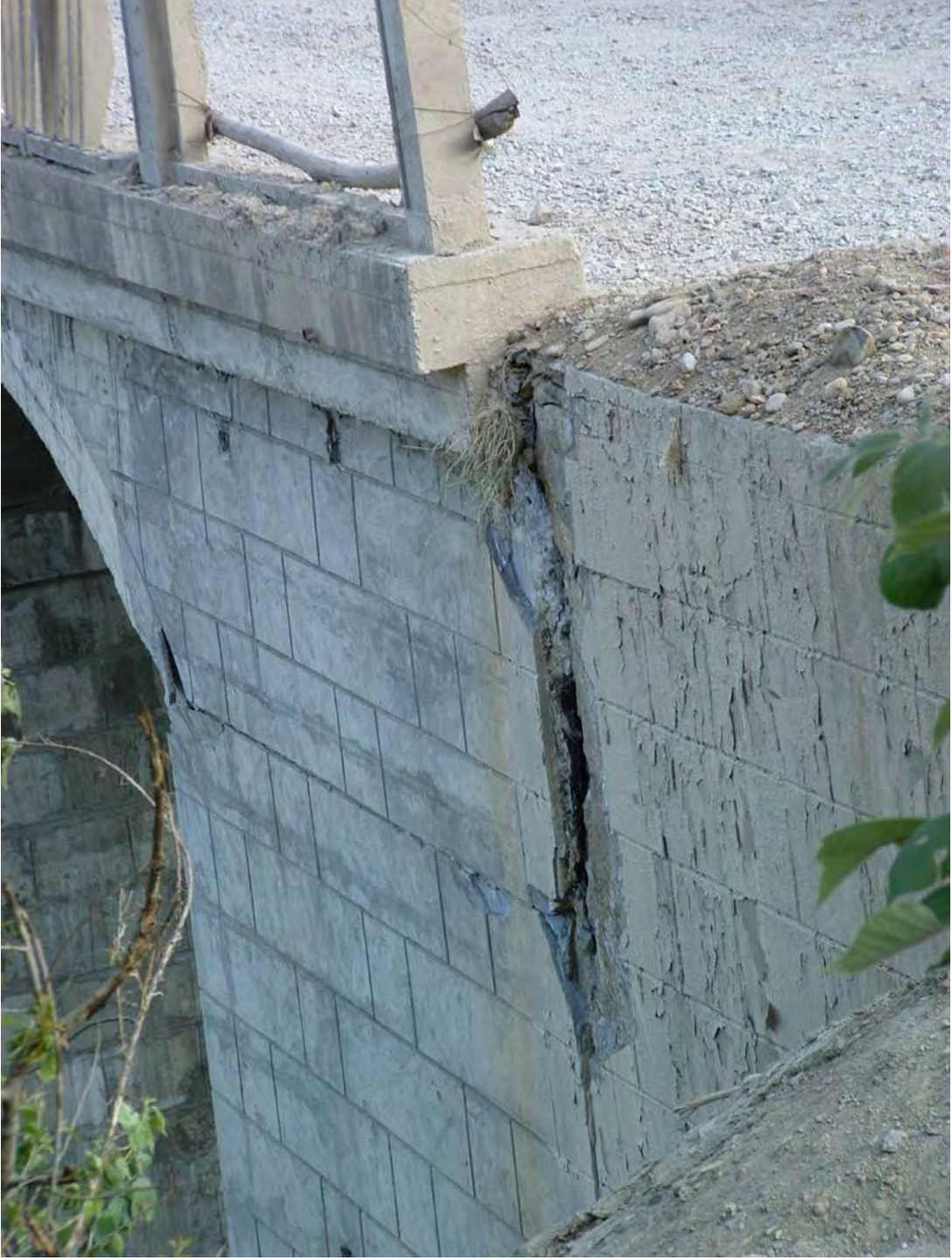
Damage to the abutment walls
