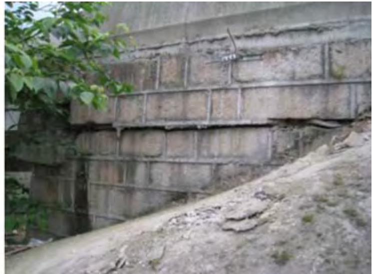
Horizontal crack and movement of the abutment wall
