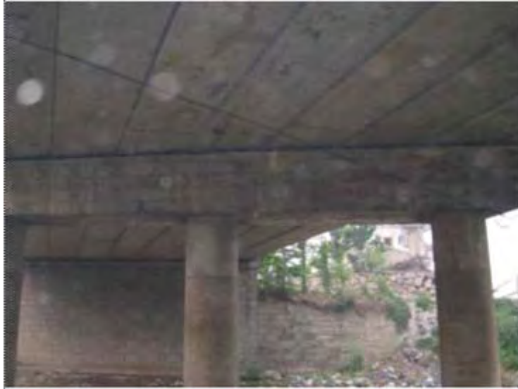
Showing the bottom of the deck which consist of precast voided concrete box girders
