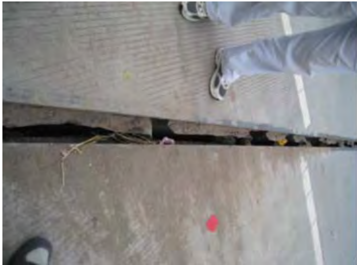
Movement of the expansion joint
