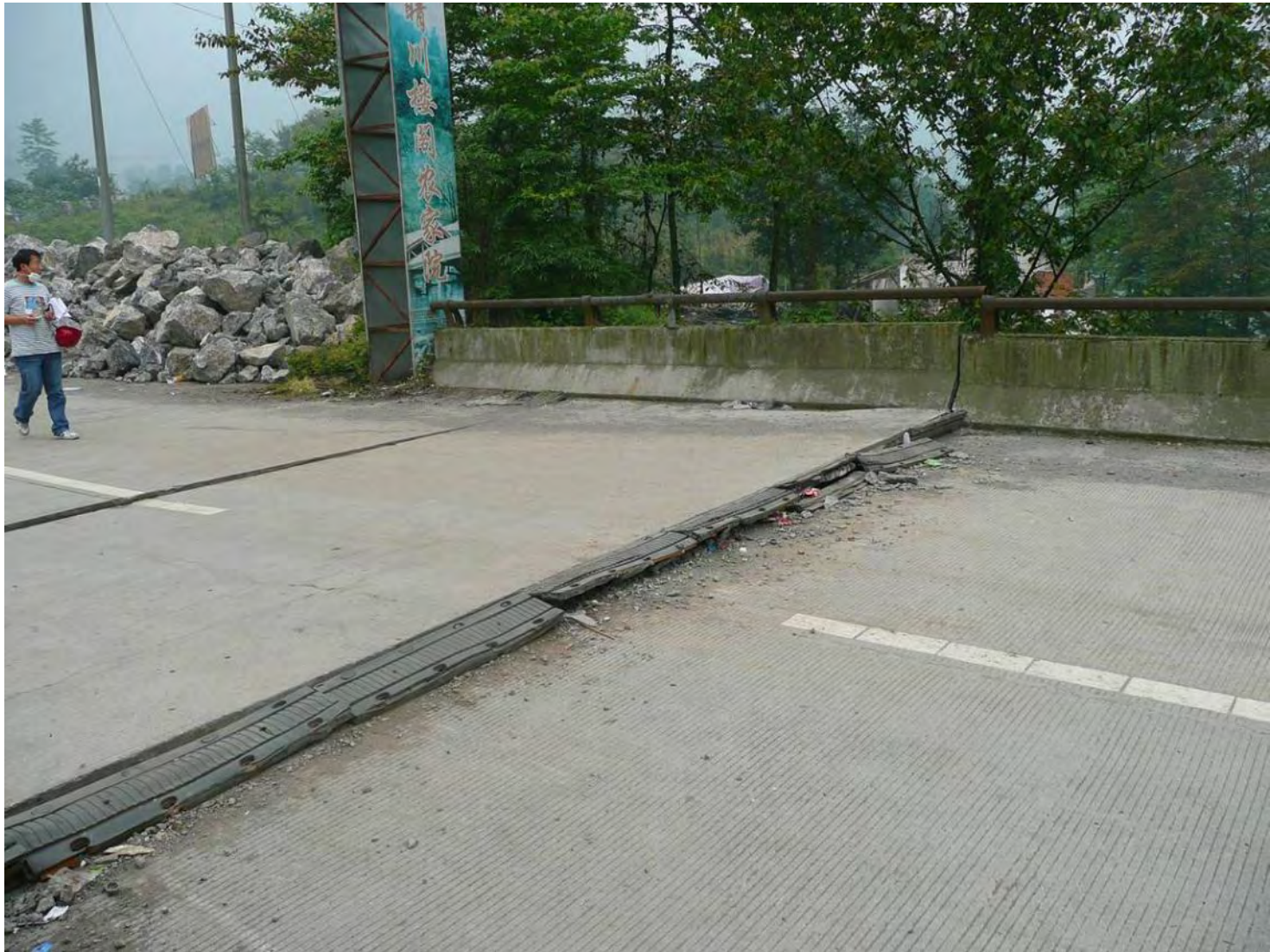
Displacement between the bridge deck and road surface at an expansion joint
