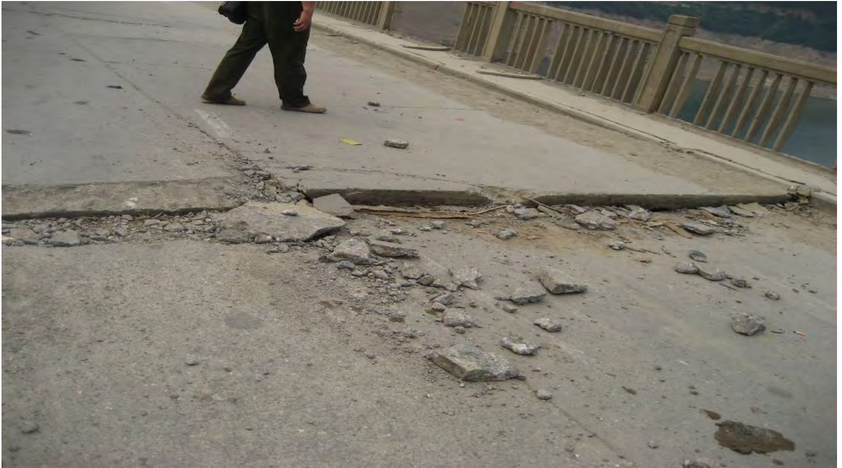
Crack in the deck
