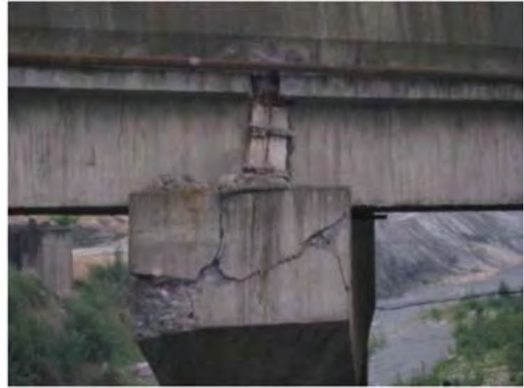
Broken pier cap
