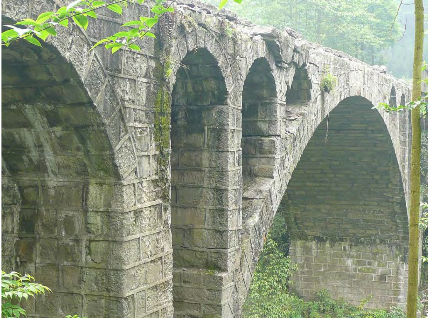
Cracks at the top of the most interior arch
