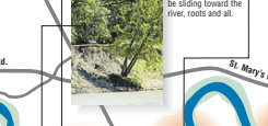
Mager Drive Riverbank erosion threatens a home just south of St. Mary's and St. Anne's roads.
